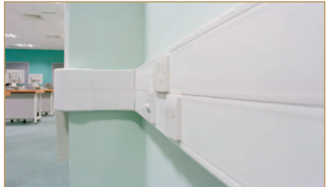
Twin Plus Trunking installed into the University of Plymouth
